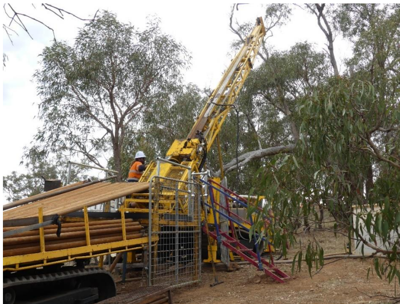
Figure 1: The diamond drilling rig on site and operating at the Nuggetty gold mine
