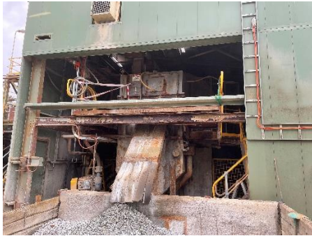
Figure 1. Old SAG discharge hopper
