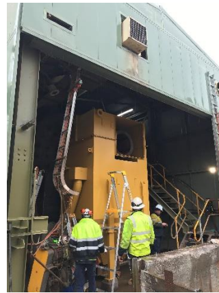
Figure 2. New SAG discharge hopper
