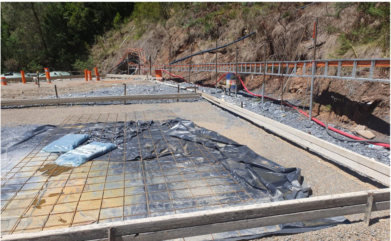
Figure 2: Generator and substation concrete pads awaiting concrete pouring and showing the orange HV cable conduits awaiting surface power generating equipment.
