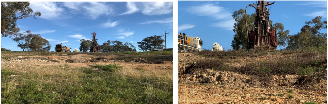
Figure 2: Drilling Rig and support truck looking across one of the backfilled historic Rockdale shafts.
